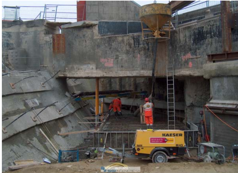
Figure 1. Worksite of the interface between Linac 4 transfer tunnel and Linac 2. The workers are close to the outer wall of Linac 2.
