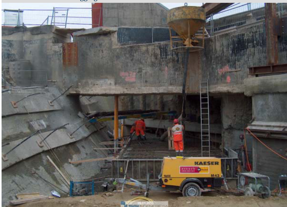
Excavating the Linac4 injector tunnel near the wall of Linac2. WP5 had to ensure that construction workers digging to the end of the tunnel would not face radiation risks.
